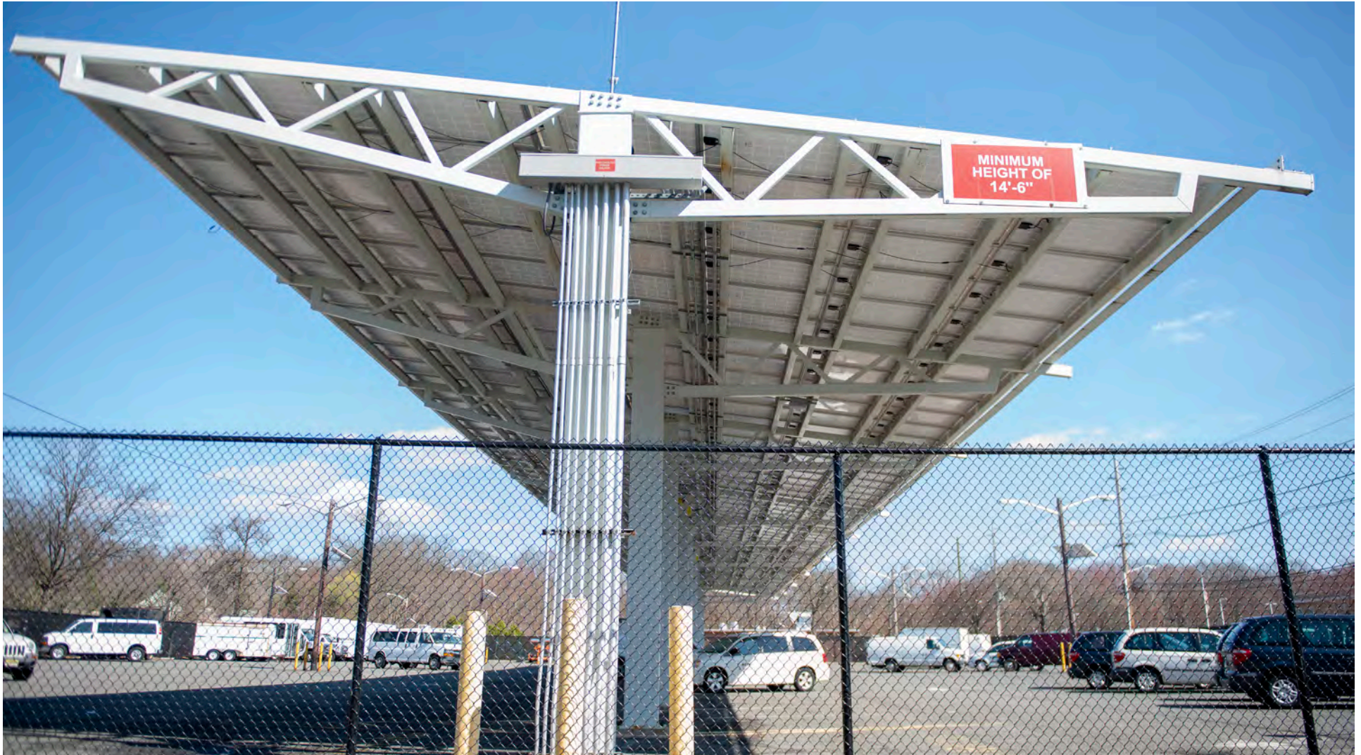
Solar Panels. Source: Donna Brennan, Bergen County
